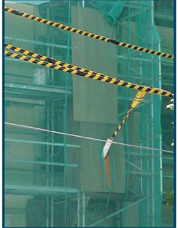
FIGURE 3 Fully enclosed energised low voltage electric lines passing through a scaffold
